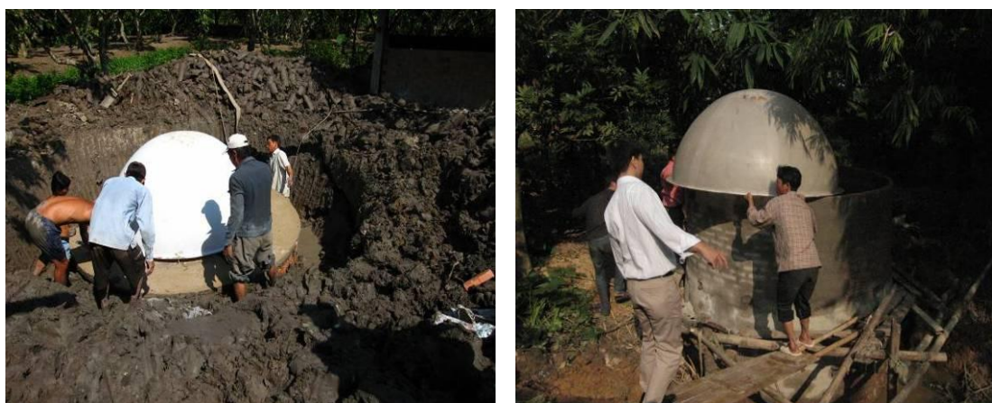
Figure VI-4: Installation of composite domes (the right for Hanoi and the left for Tien Giang)
