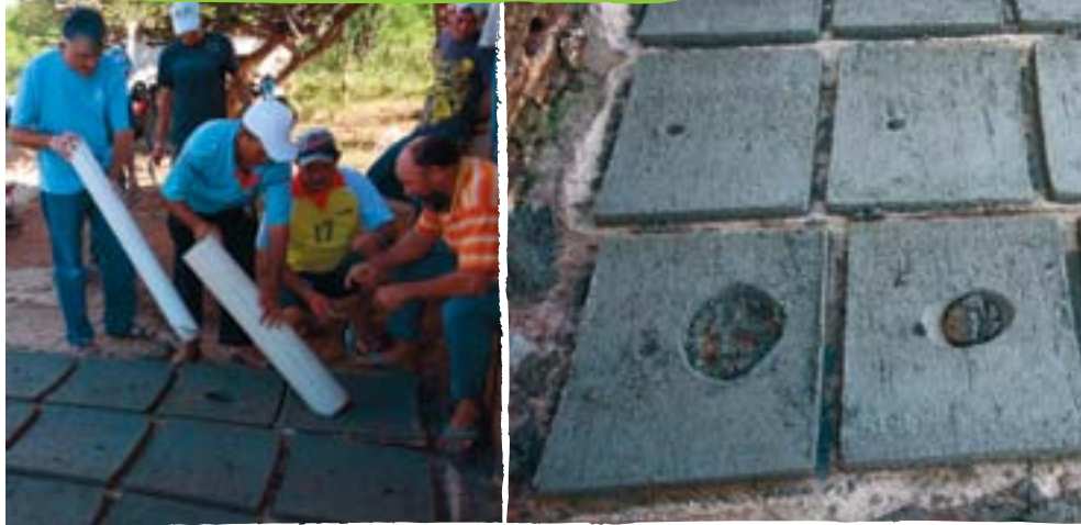
[Figure 6] Preparation of the entrance and exit holes for the input and output pipes
