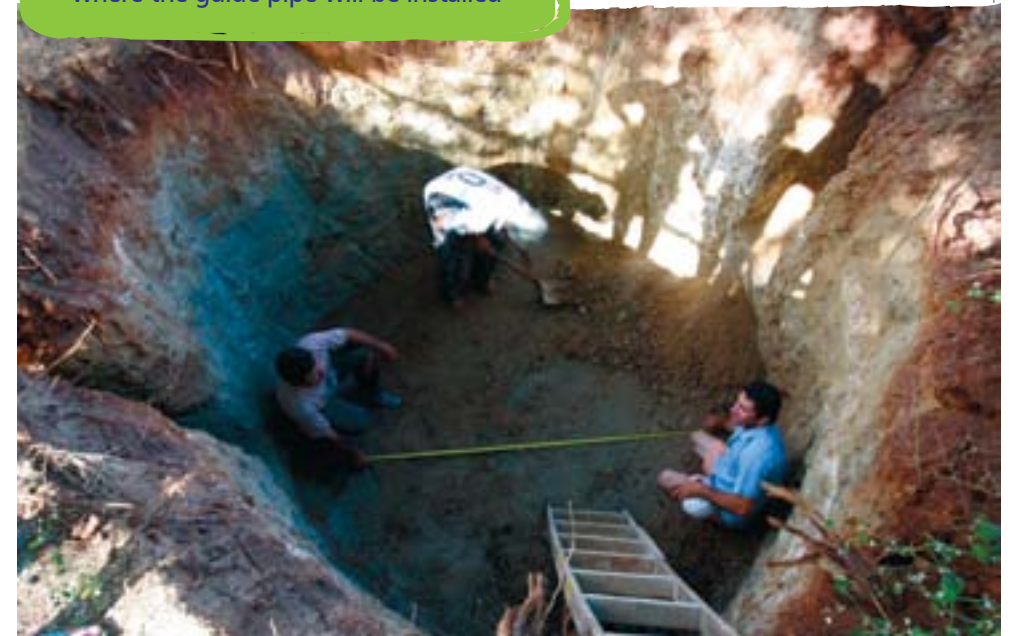
[Figure 8] Marking out the centre where the guide pipe will be installed
