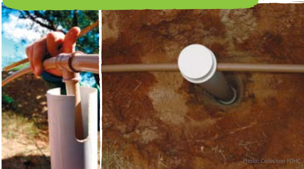
[Figure 42] Assembling and installing the drain at the gas pipe's lowest point. Notice also Figure 39
